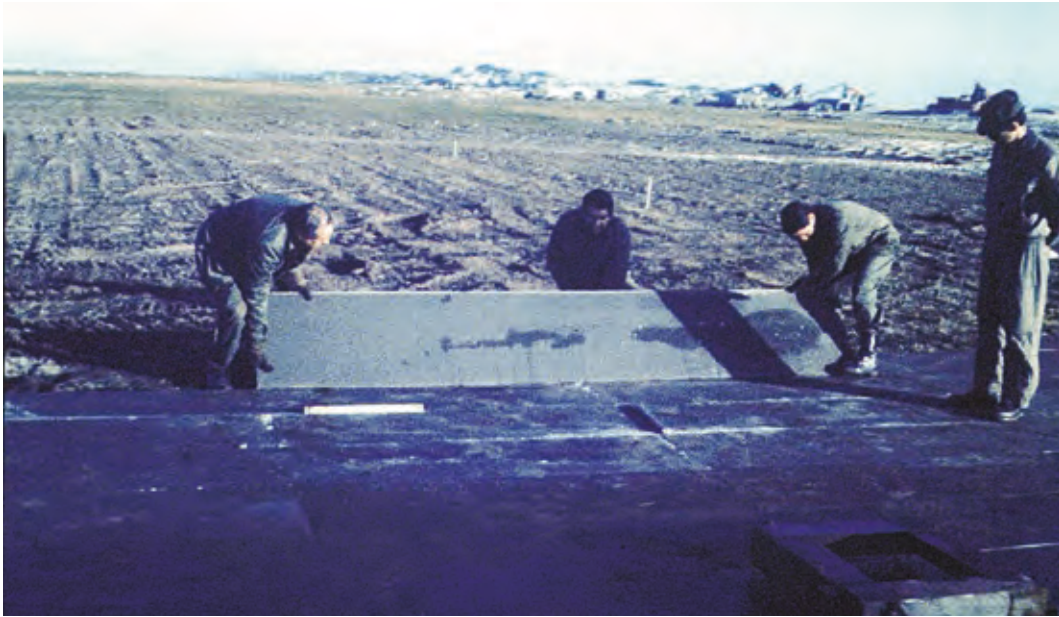
Installation of aluminum plates at BAM Malvinas - Photo courtesy of: Com. VGM (R) Grünert
