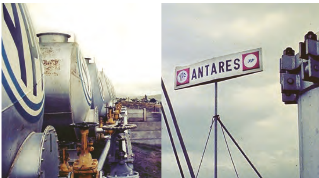
Fuel plant established by YPF Antares - Photo courtesy of: Brig. VGM (R) Bloomer Reeve
